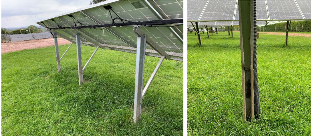
Cabling Along Panels
